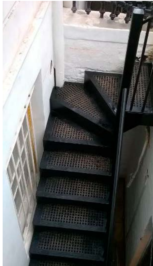
LCC Kited Staircase
